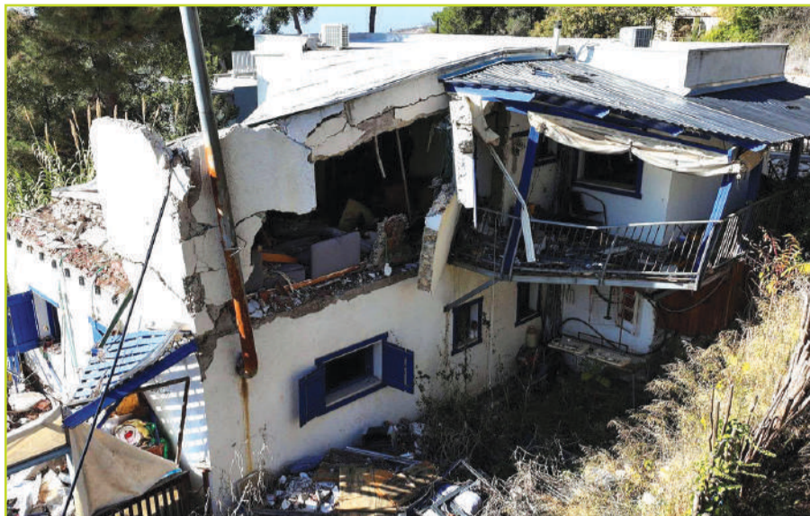
A damaged building in Kibbutz Manara, near the Israel-Lebanon border
